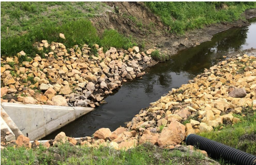
Figure 6: Le Sueur & Rice Joint County Ditch 54 riprap erosion control, June 22, 2020
